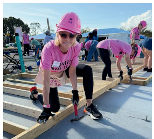
ABOVE: Supervisor Leslie Swan hammers nails into a frame at Habitat for Humanity's 2026 Women Build on March 7. AT LEFT: Voter Services Manager Katherine Bauman stands on a ladder as she prepares to hammer nails into a frame.
